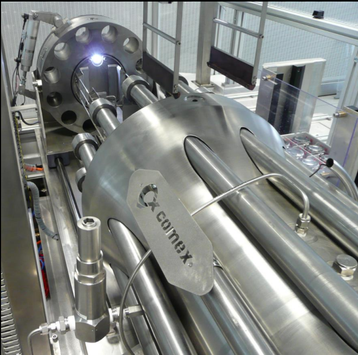
Development and on-site installation of a test facility for ROLEX watches (600bar) including control by camera. (image courtesy: ROLEX)
